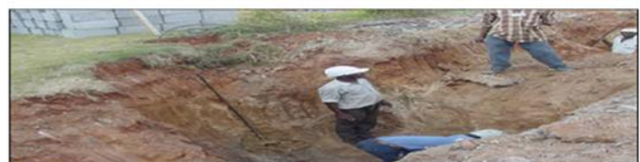
Pit without Barrication
