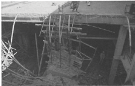
A Formwork Failure
