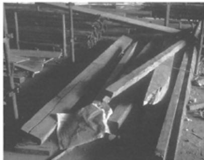
Damaged Formwork Materials
